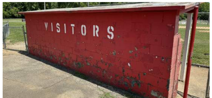
Flood damage to the dugout at Babe Ruth Sports Complex
